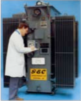
(a) 1000 kVA oil-immersed
